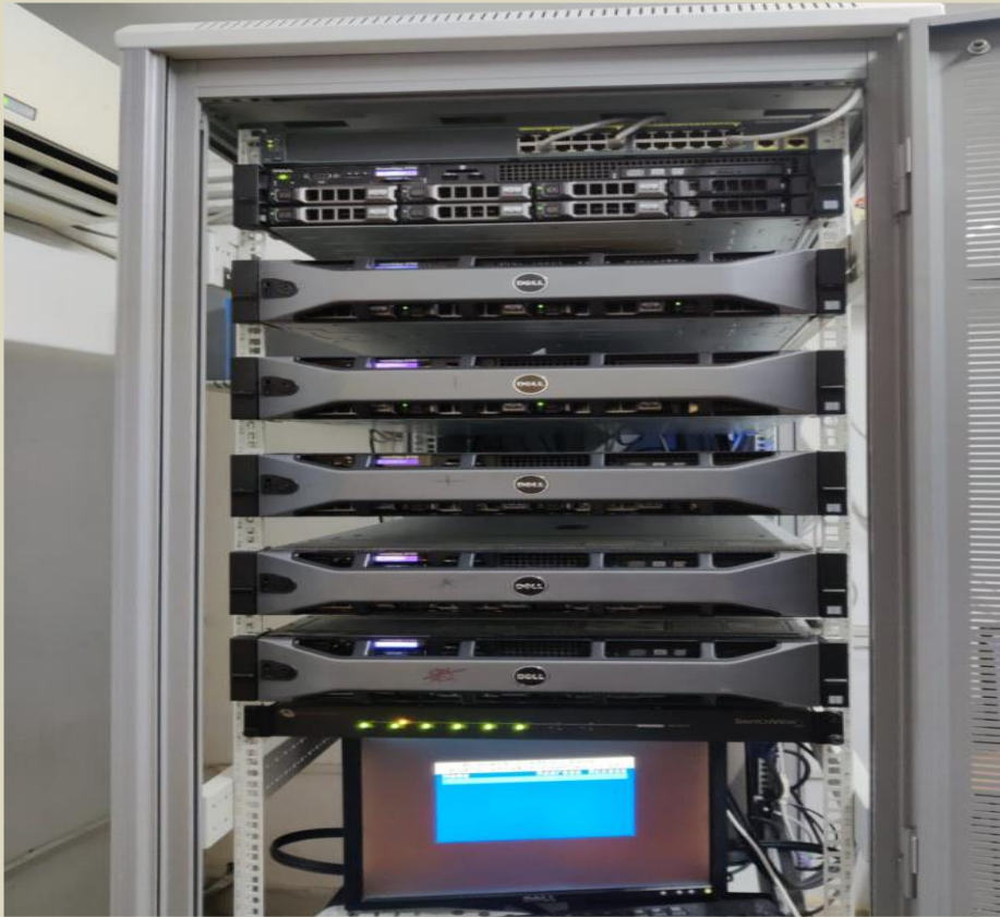
WEBSERVER, AUTHENTICATION SERVER and OTHER SERVERS HOSTED IN SERVER ROOM (Room No.G04, Ground Floor, SIT)
