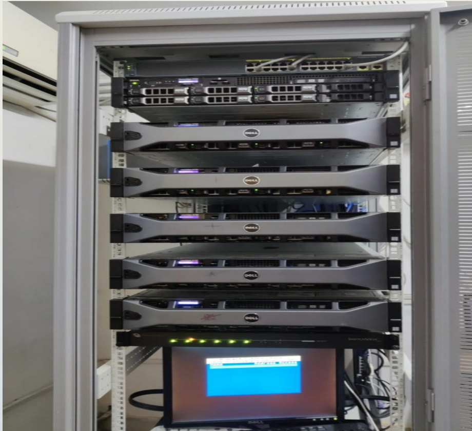
WEBSERVER, AUTHENTICATION SERVER and OTHER SERVERS HOSTED IN SERVER ROOM (Room No.G04, Ground Floor, SIT)
